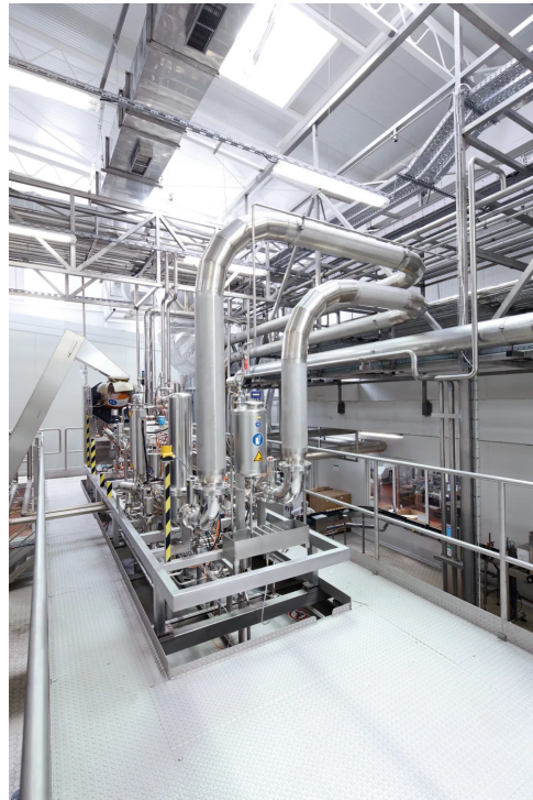
↑ The roof of the block also serves as the filler's service module with easy access to the maintenance area.
